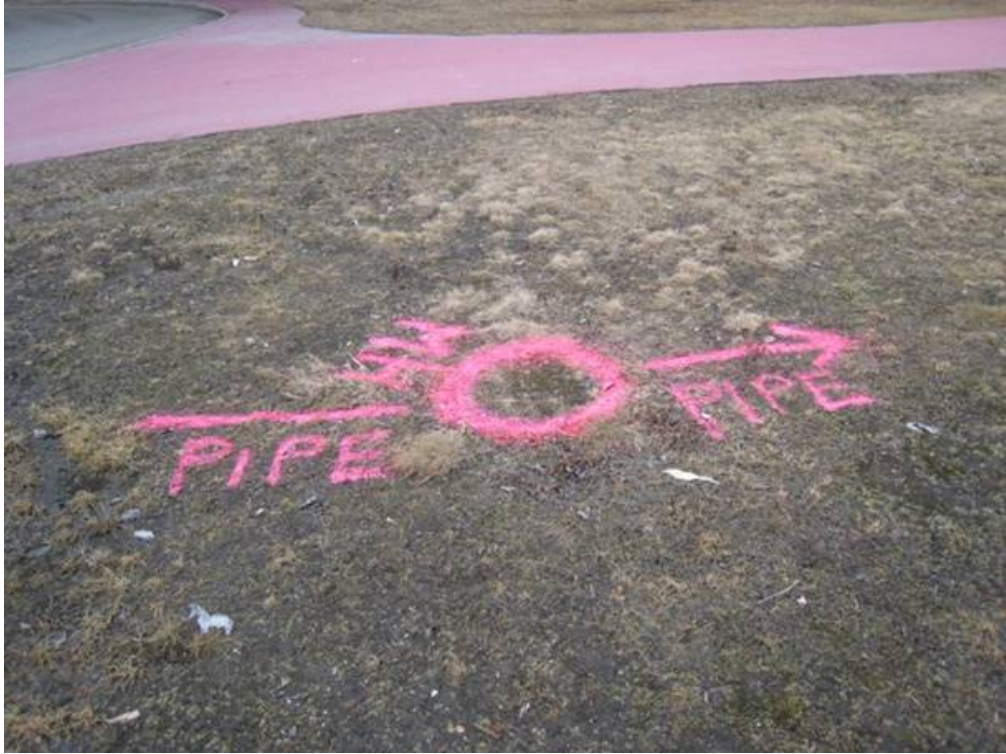
Close-up View of Centreline of City Underground Pipe at NE Area of Site.
